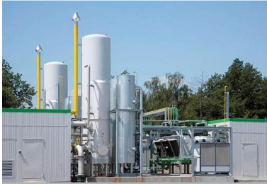
Biogas Plant of Mühlacker
